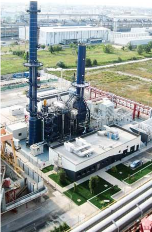
Enel hydrogen power plant in Fusina, Italy.
